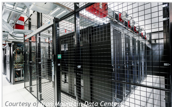
Courtesy of Iron Mountain Data Centers
